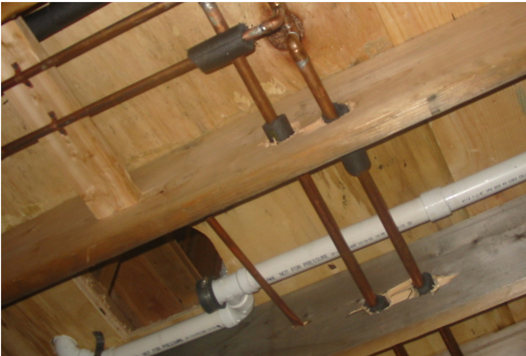
Acceptable - Bored holes less than than 1/3 of joist
