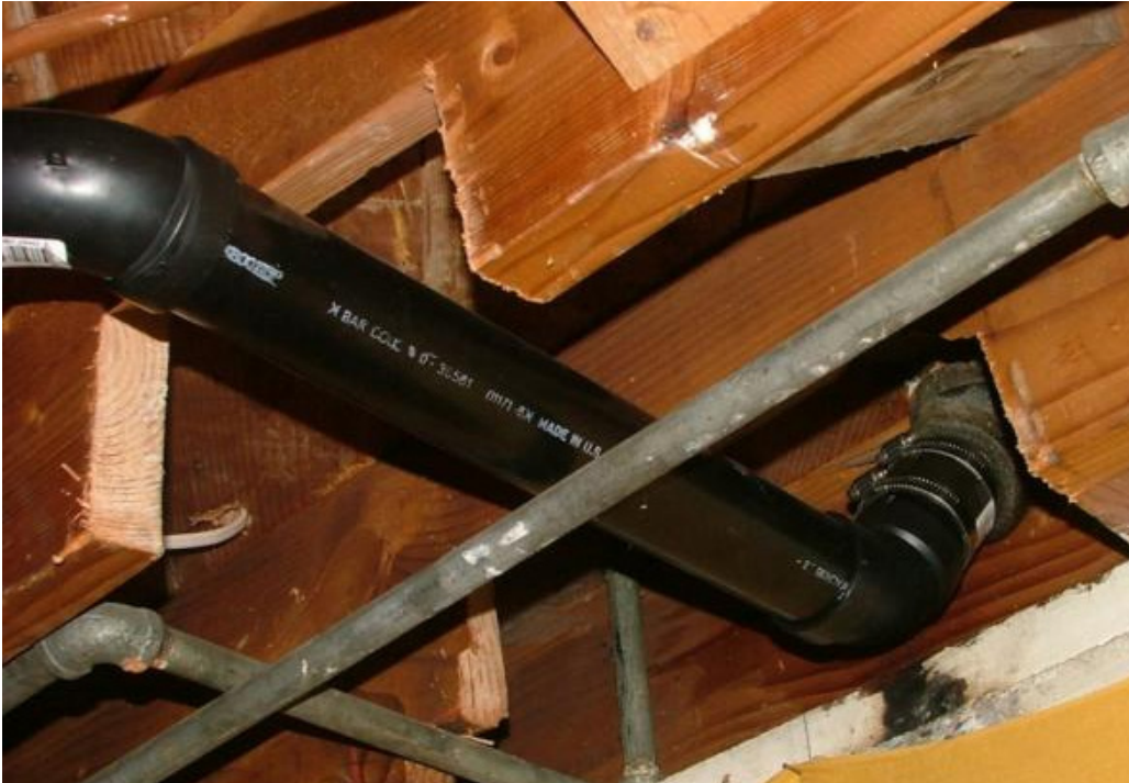
Not Acceptable - Notch greater than 1/6 of joist
