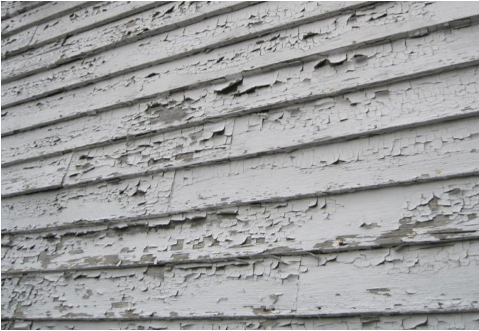
Flaking Lead Paint on Wood Siding
