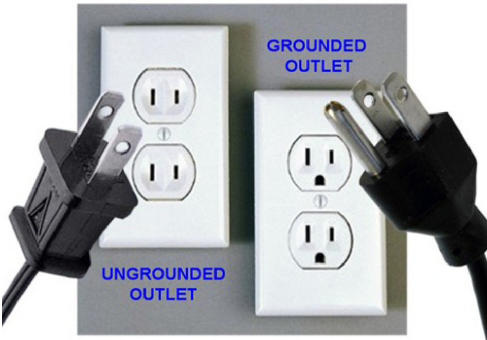
Ungrounded outlets will often need to be replaced with grounded outlets which requires rewiring all the way to panel
