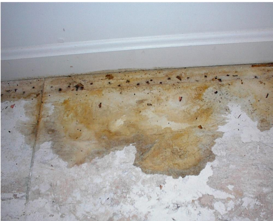
Pet / Animal Damage at Subfloor
