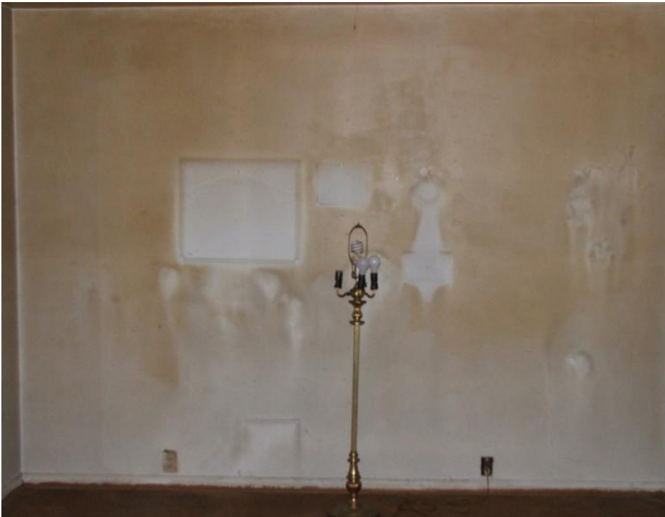
Nicotine Damage to Interior Walls
