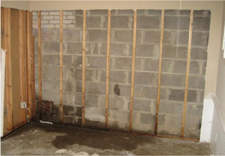
Rotten wood bottom plate at basement water infiltration
