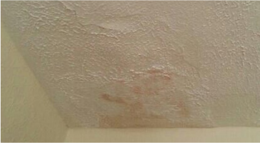
Water damage at ceiling from roof or plumbing leak
